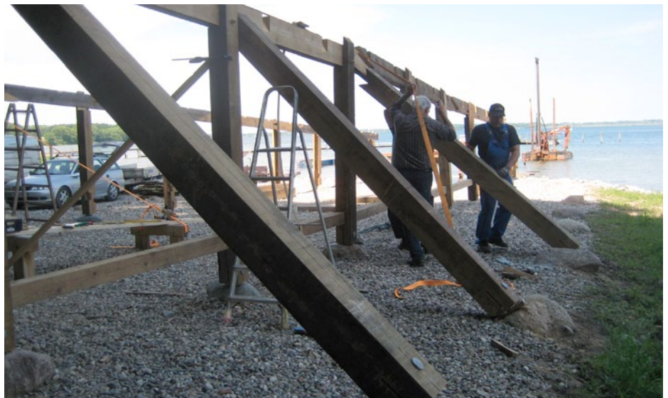
The ship shed (or 'naust') being built on the shores of Allsund, Denmark, to house the reconstruction of the 4th century Nydam ship.
